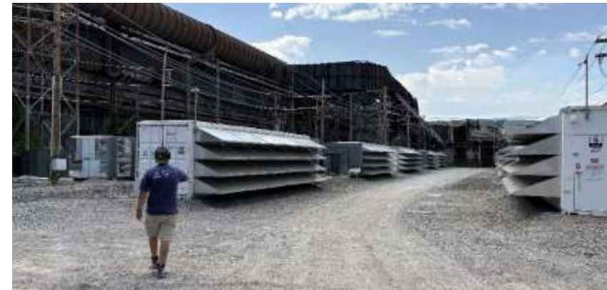
Above: Canaan's hosted miners in Midland, PA Operated by Mawson Infrastructure Group
